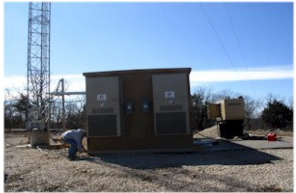
KSEF Transmitter Site in Park Hills, Missouri
